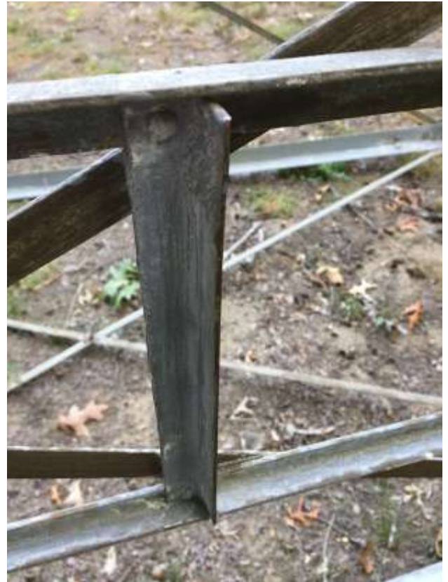
Unsafe to Climb?
