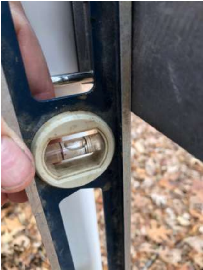
Figure 2: Make the Boom-to-Mast Plate Plumb (I pulled the level away as I snapped the photo, but the bubble should be in the center.)
